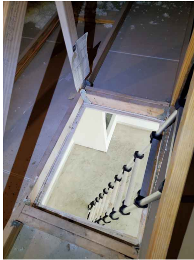
Viewed From: Decked Areas of Attic Approximate Average Depth of Insulation: 12 Inches
