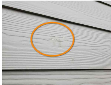
Right Side (Damaged)
