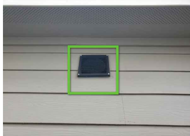
AC Fresh Air Intake
