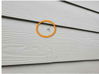
Left Side (Damaged)
