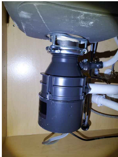
General Images Of Range Hood/Exhaust System :
